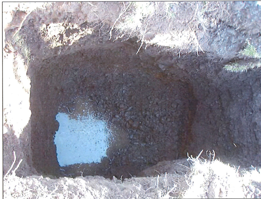
Photo 2: Groundwater Seepage in Test Pit TP3
