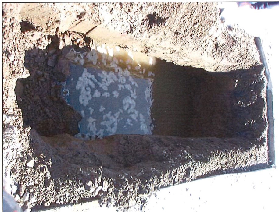
Photo 4: Groundwater Seepage and Gravel Deposits Cave-In in TP8
