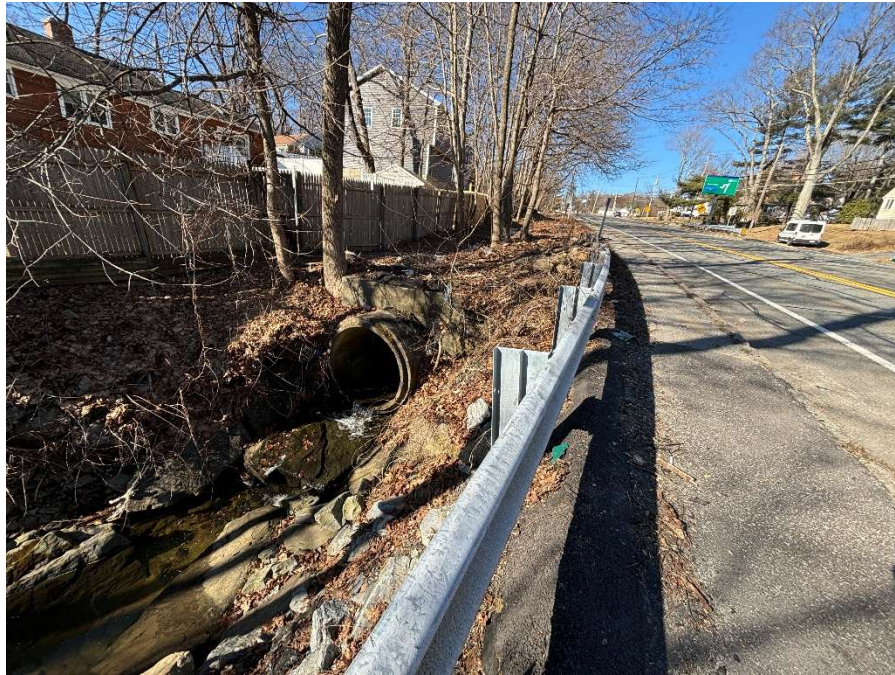
Photo 4. Upstream (westerly) view of D-Series stream flowing out of pipied conveyance.
