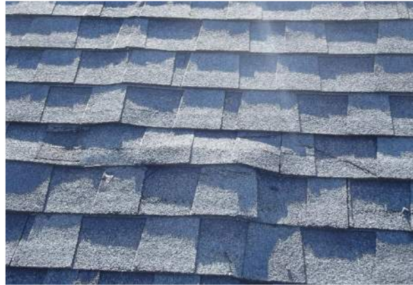
Photo 8 – Bulge in roof deck.
