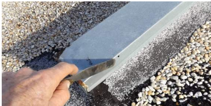
Photo 16 – Abandoned rail curb. Metal cap is not secured.
