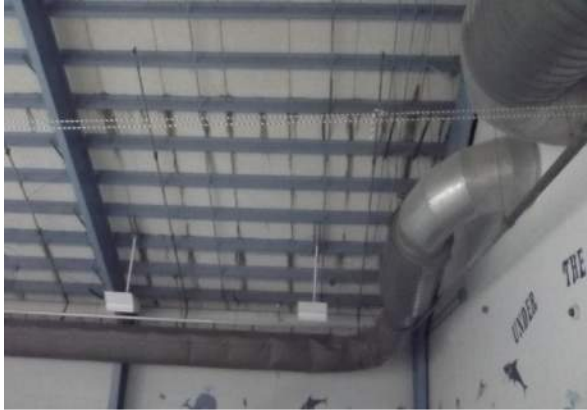
Photo 7 – Staining on tectum deck.
