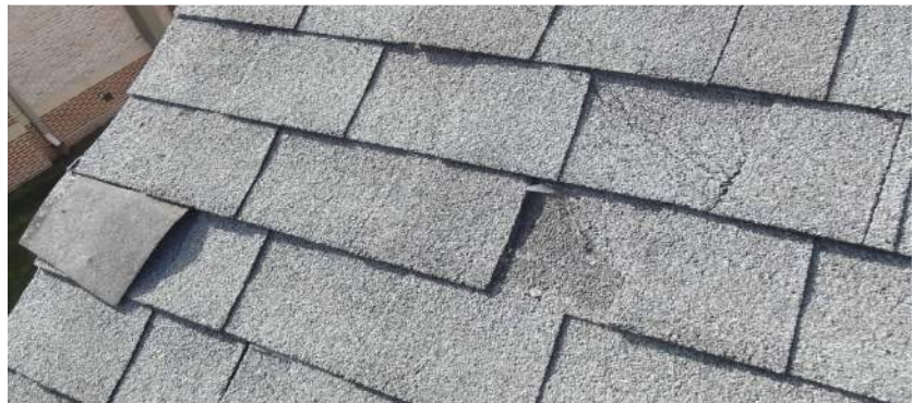
Photo 14 – Loose shingles at dormer.
