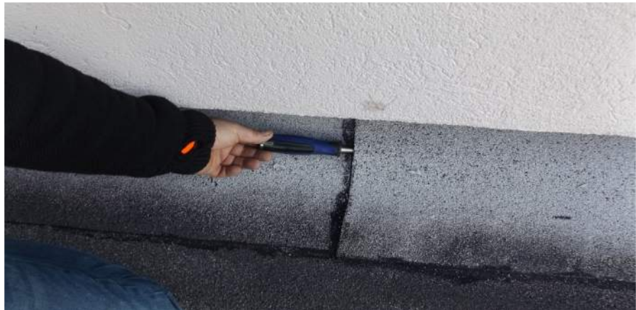
Photo 21 – Opening in flashing at rising wall.
