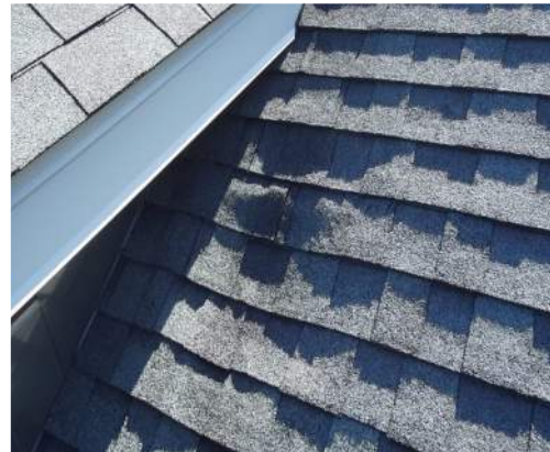
Photo 2 – Roof deflection below dormer valley.
