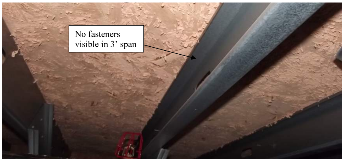
Photo 6 – Missing fasteners in plywood.
