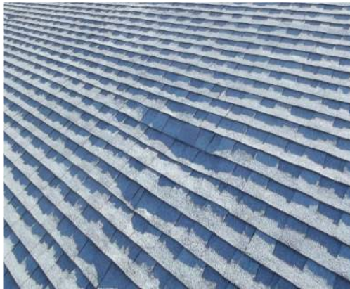
Photo 1 – Roof deck deflection in field of roof.
