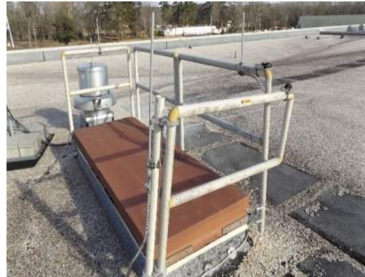
Photo 18 – The fall protection rails around the hatch units are deteriorating.
