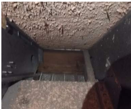
Photo 3 – Fireproofing delaminating from plywood.
