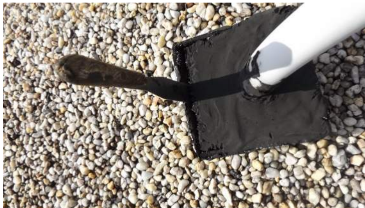
Photo 15 – Deterioration at pitch pocket. Typical condition
