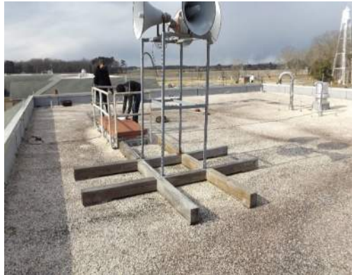
Photo 17 – Wood base of speaker system is not on a slip sheet.
