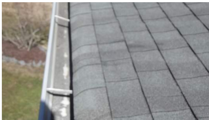
Photo 11 - Shingles curling down into gutter.
