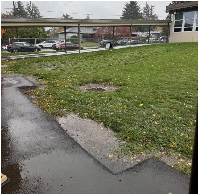
Site where flooding occurs during downfall
