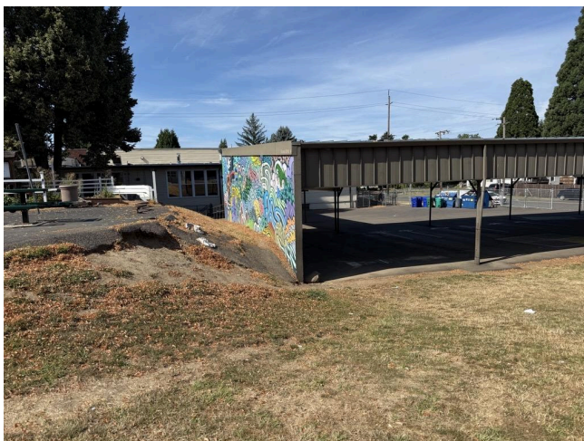
East Covered Space, retaining wall, steep slope, broken asphalt slab
