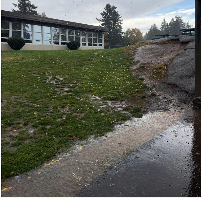
Slope condition near Annex building and East Covered Space, trench drain (to be rain garden)
